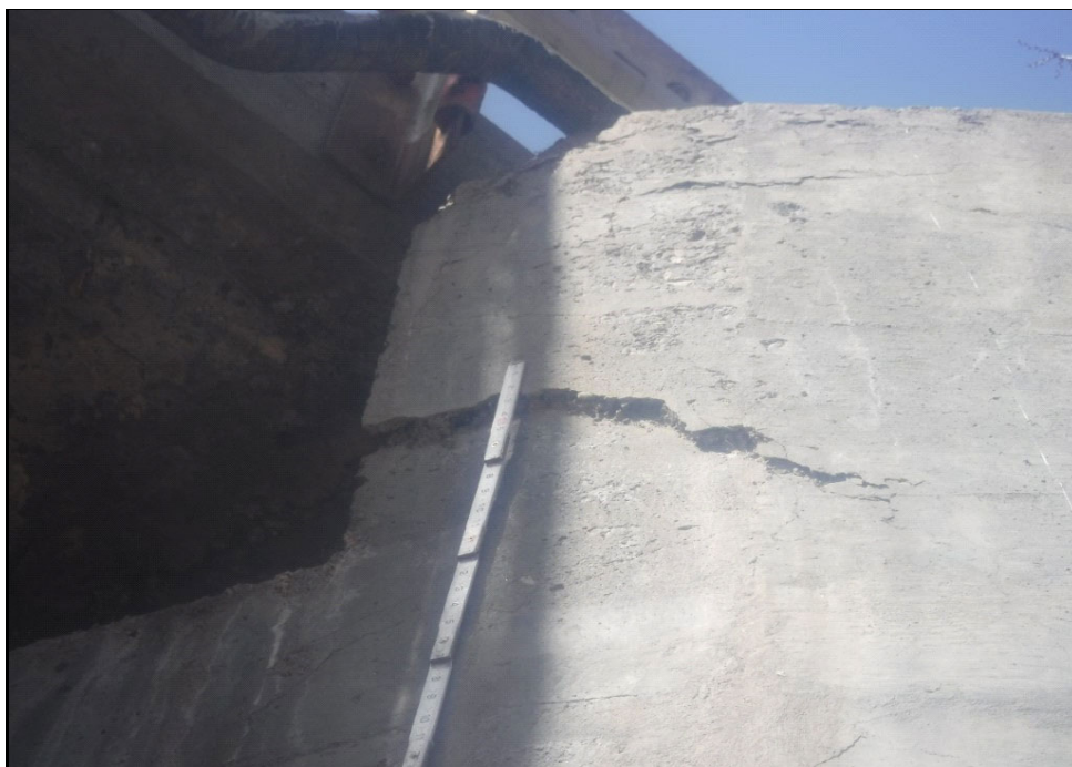
Wide horizontal crack in northeast wingwall
