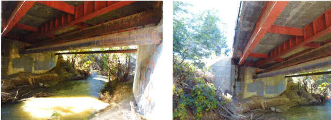
Photographs show the Little Salt Wash, the underside of the bridge, and general abutment conditions.
