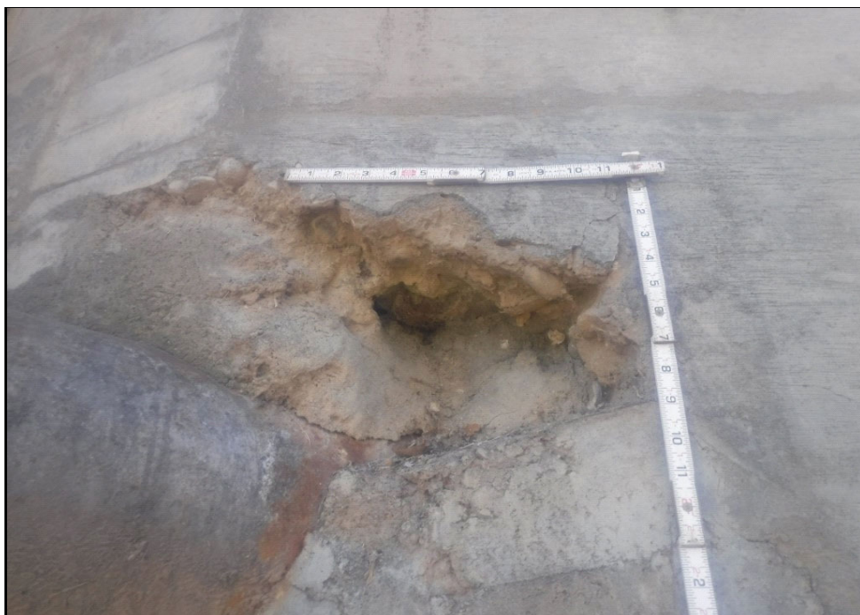
Spall in southwest wingwall at utility
