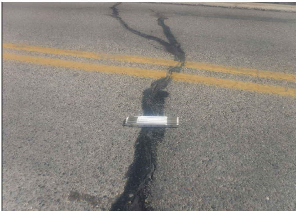
Sealed transverse crack in asphalt at back face of Abutment 2 reopening
