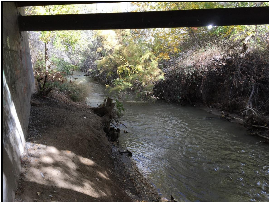
Photo 2. Representative image of the north creek bank below the existing Maple Street Bridge crossing. View is to the east.
