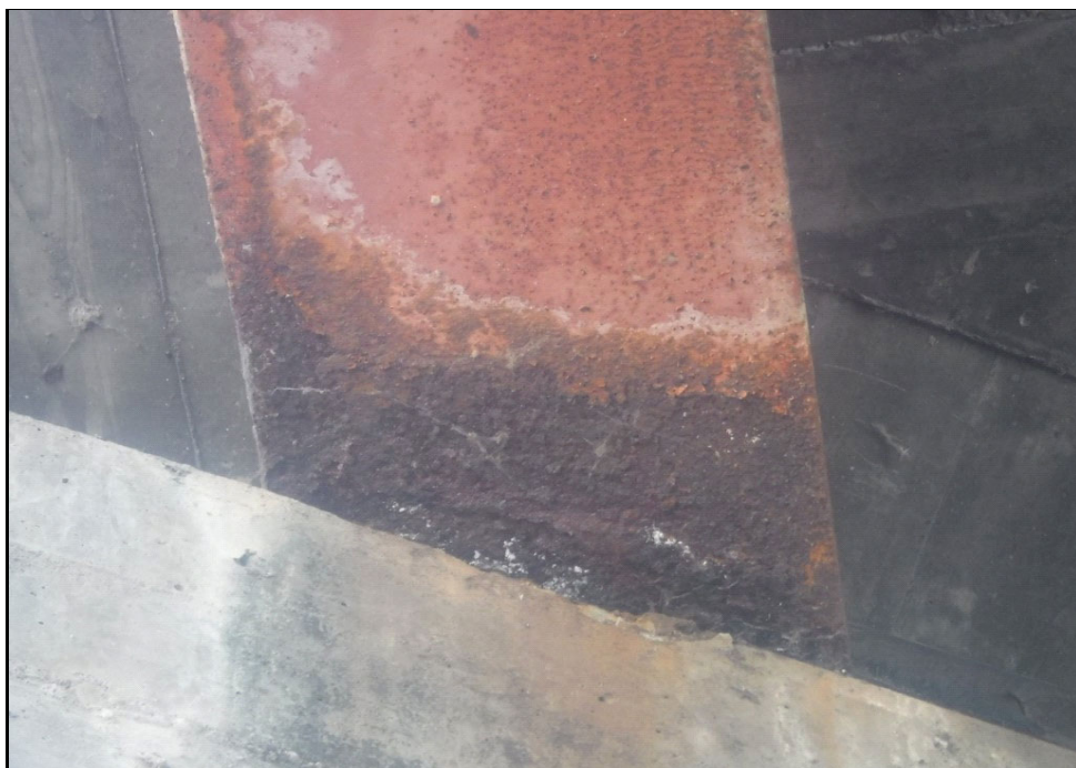
R2 rust of bottom flange of Girder D at Abutment 1
