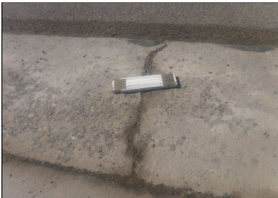
Wide transverse crack in west sidewalk
