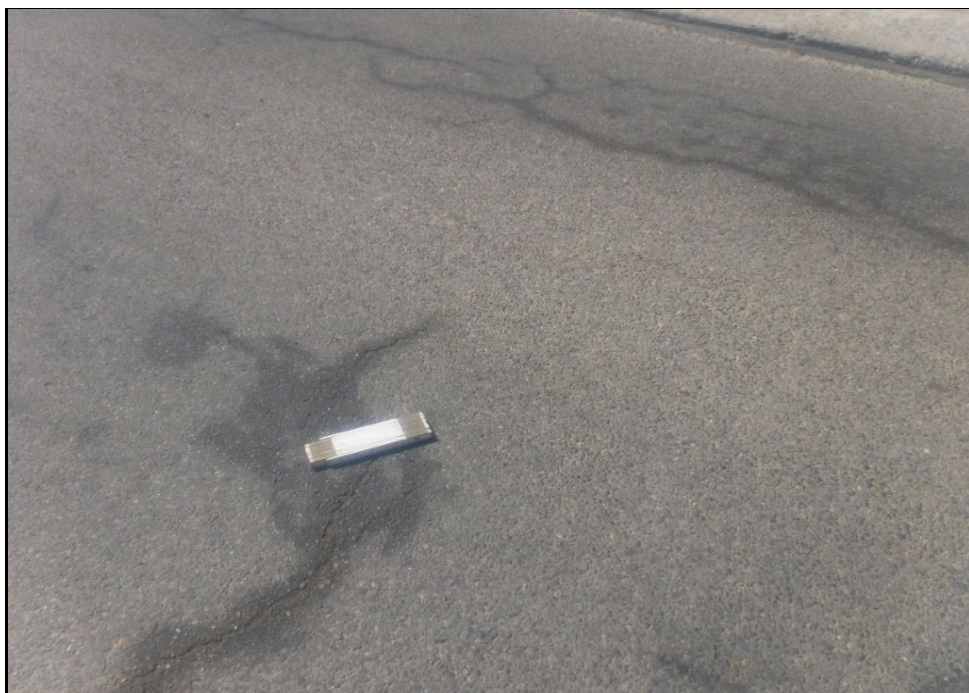
Transverse and longitudinal cracks in asphalt on deck
