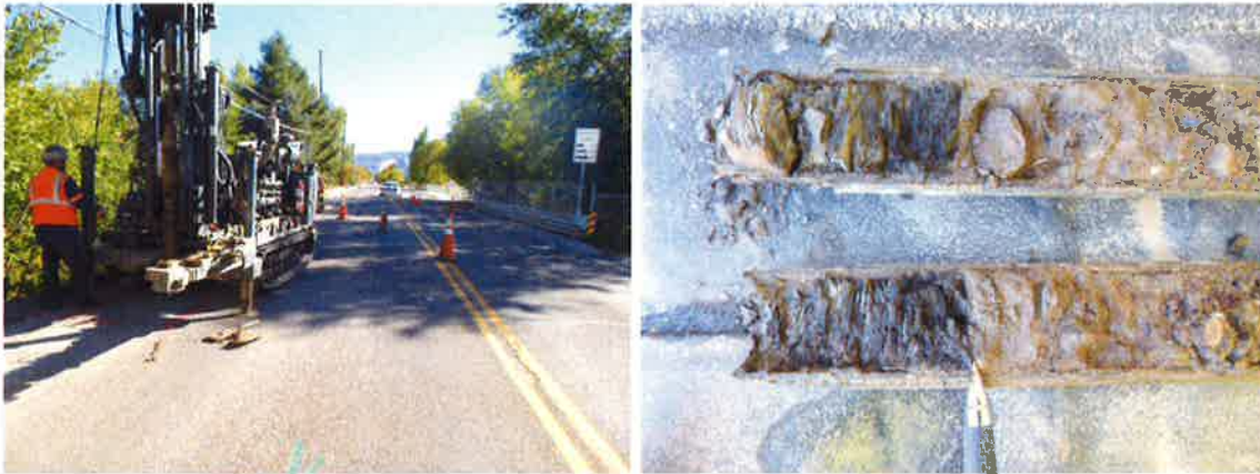
Left Photograph showing drill rig at the BH#2 site, view to the south. Right photograph showing contact between overlying sand/gravels (right of the pen) and shale (left of the pen) in BH#1 at about 61 feet below grade.
