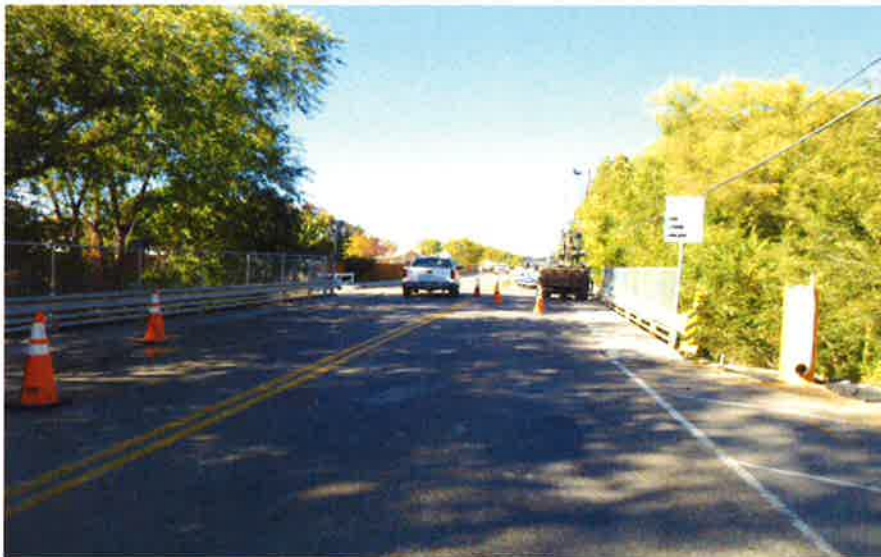
Looking north showing the existing bridge deck with drill rig positioned at the location of BH#2 near the north abutment.
