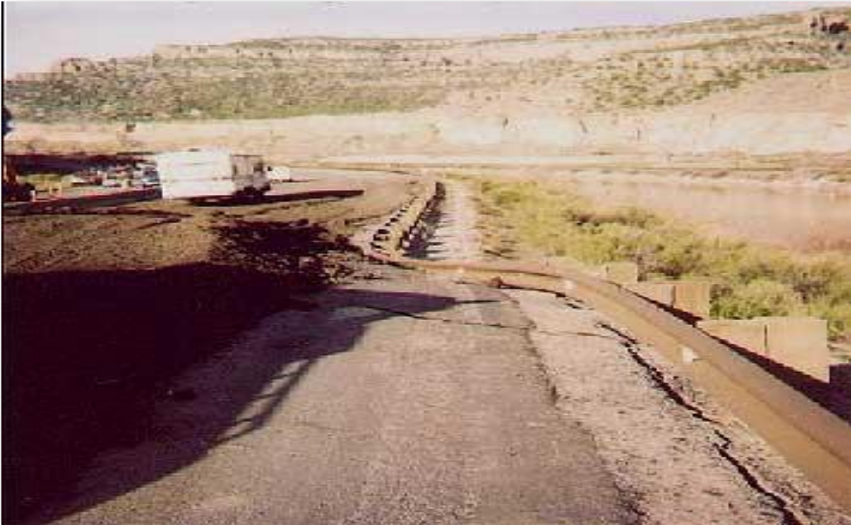
FIGURE 11 PHOTO OF DEBEQUE CANYON SLIDE AREA- INTERSTATE 70
