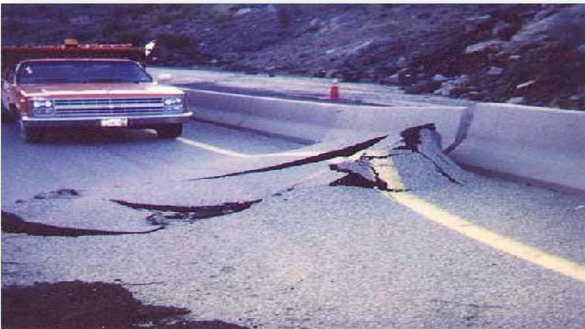
FIGURE 12 PHOTO OF DEBEQUE CANYON SLIDE AREA- INTERSTATE 70
