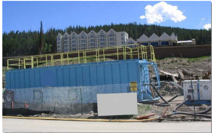
Photograph CT-1. Proprietary chemical treatment system being used on a construction site with sensitive receiving waters. Photo courtesy of WWE.
